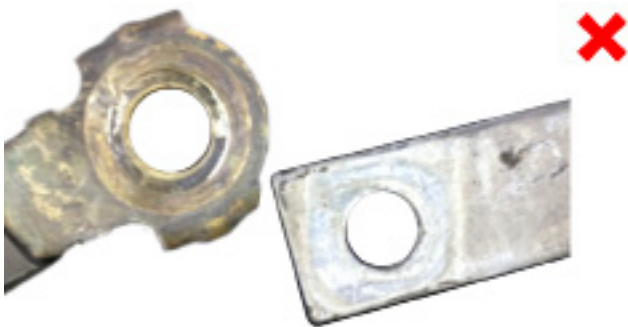
Fig. 1. Ground connection prior to cleaning: Poor connection
