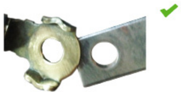
Fig. 2. Ground connection following cleaning: Good connection
